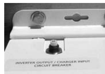
Circuit Breaker Reset
