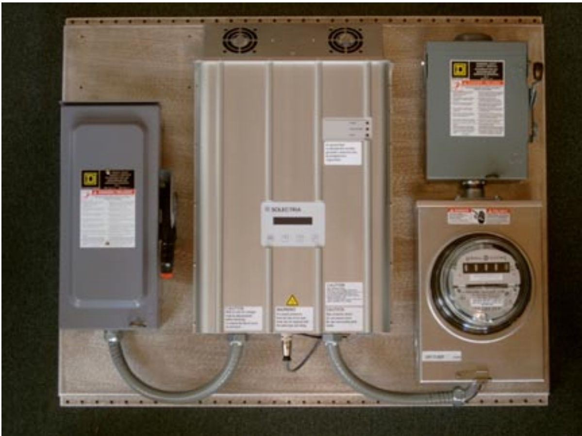
Fig. 7 A typical PVI 1800 or PVI 2500 installation with AC and DC disconnects. (AC disconnect is on the right, DC disconnect on the left. PVI 2500 shown.)
