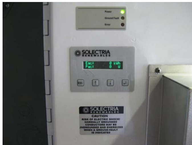
Fig. 7 Front view of inverter showing LED indicators, LCD display and ground fault warning label
